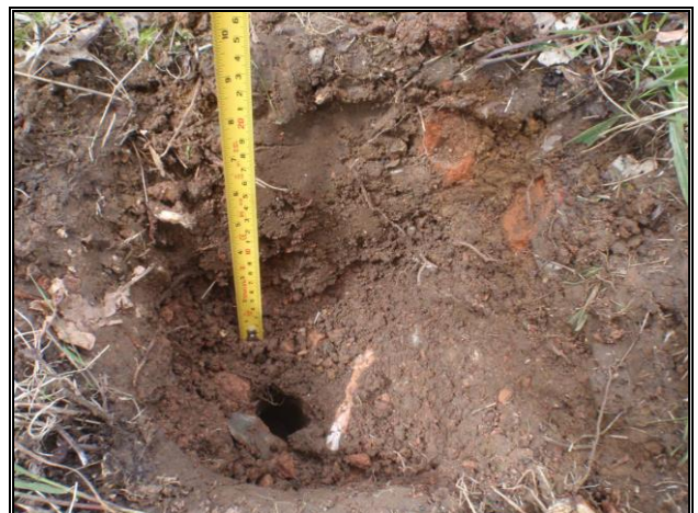
Plate 23 : Soil Profile 3 showing brick fragments at TH37
